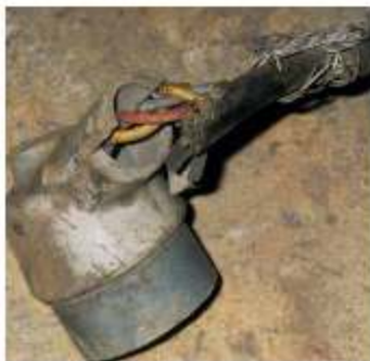
Damaged cable grip
