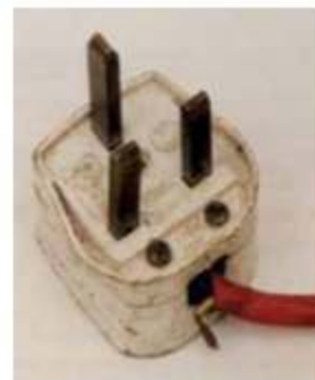
Damaged cable sheath
